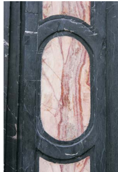
Fig. 8. A fragment of the portal of the St. Adalbert Church made of the black Dębnik limestone with a marquetry of the Paczółtowiec limestone. The church, about 1000 years old, is one of the oldest in Cracow; its late Baroque portal comes from the 18 th century
