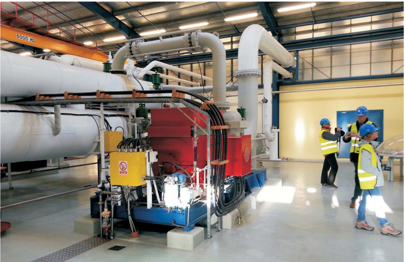
Ryc. 4. Turbina i generator o mocy 1,2 \text{ MW}_{el} , turbina jest napędzana wodą o temperaturze ok. 95^{\circ}\text{C} . Obie fot. L. Pająk Fig. 4. The ORC turbine and generator with a capacity of 1.2 \text{ MW}_{el} are showed below, the turbine is driven by a water with temperature of ca. 95^{\circ}\text{C} . Both photos by L. Pająk
