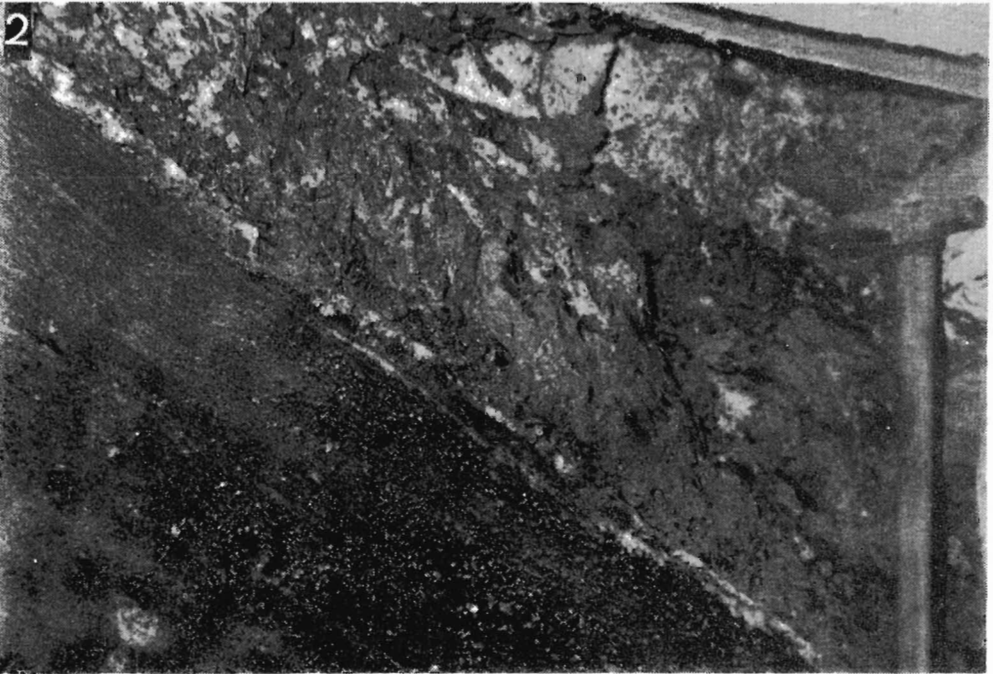
1 — Uppermost part of the Stratified Salt Member and its contact with the Salt Breccia Member in the northern part of the Wieliczka Mine; Kaniów Gallery ( photo by W. ZALEŃSKI ) 2 — Similar situation in Rarańcza Gallery ( photo by W. ZALEŃSKI )
