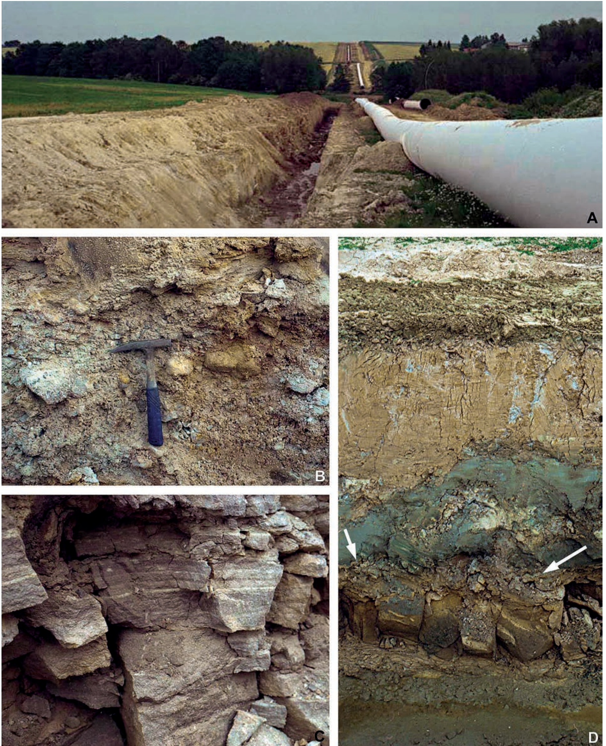
Text-fig. 4. Field aspects during excavations for the OPAL pipeline in the Dittmannsdorf area in 2011. A – trench of the OPAL pipeline north of Niederschöna (view towards the northeast). In the foreground, fluvial strata of the Niederschöna Formation are exposed; in the background (behind the wooded belt), Proterozoic gneiss crops out capped by a red-weathered palaeosol (caused by pre-Cenomanian “Rotlehm-Verwitterung”). B – lower part of the fluvial Niederschöna Formation consisting of coarse-grained pebbly sandstones with conglomerate lenses (so-called “Grundschotter”). C – cross-bedded fluvial sandstones of the Niederschöna Formation up-section of the Grundschotter. D – detail of the OPAL pipeline trench 2.5 km northwest of Haida showing the contact of the Niederschöna Formation below and a basal greensand of the Mobschatz Formation above (arrows); the uppermost part of the section is composed of Quaternary loess
